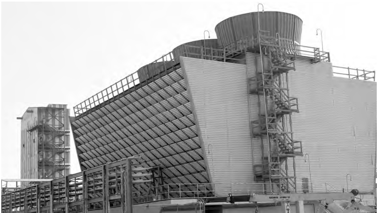
State-of-the-art Nitric Acid plant, Dahej
