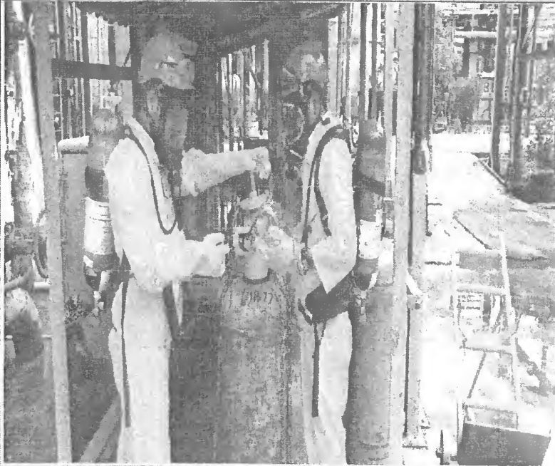
Emergency crew members applied kit on the leaky cylinder
