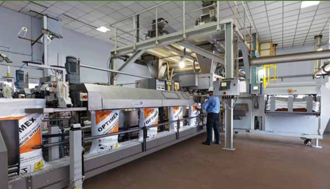
TAN bagging plant at Taloja
